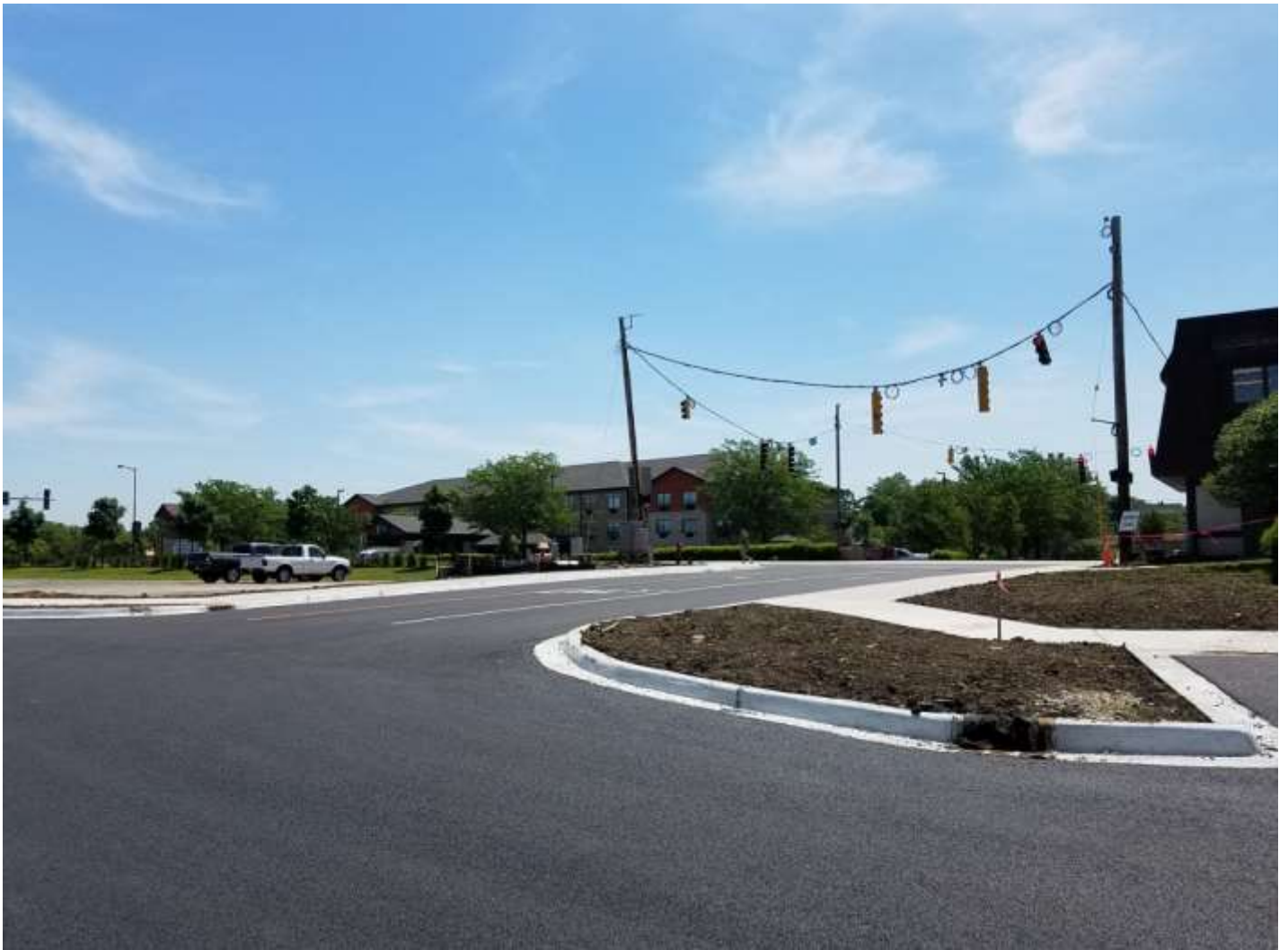
Stage 1- Completion of Spring Street Drive, north of Aurora Township Bldg. 06/07/2018, looking NE.
