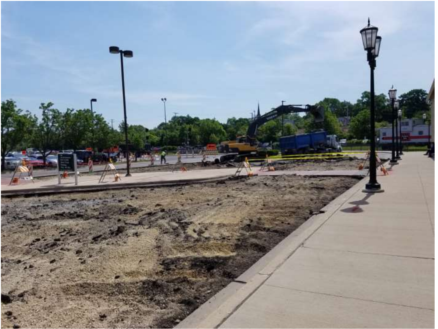
Stage 2 Work -Excavation and Pavement Removal at ATC Parking Lot-north of ATC Building 06/07/2018
