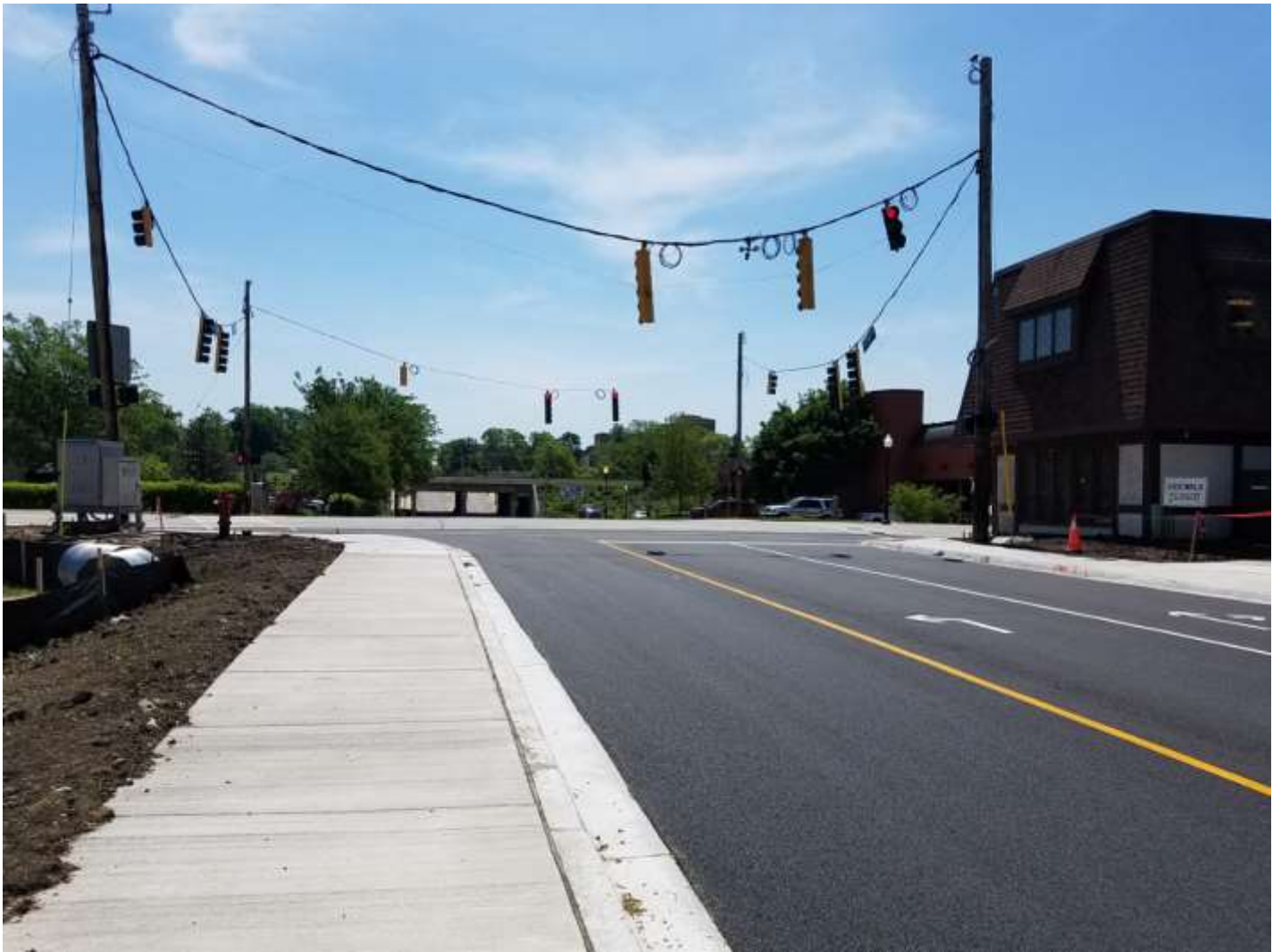
Stage 1- Spring Street Drive, entrance north of Aurora Township Bldg. 06/07/2018. Looking East.
