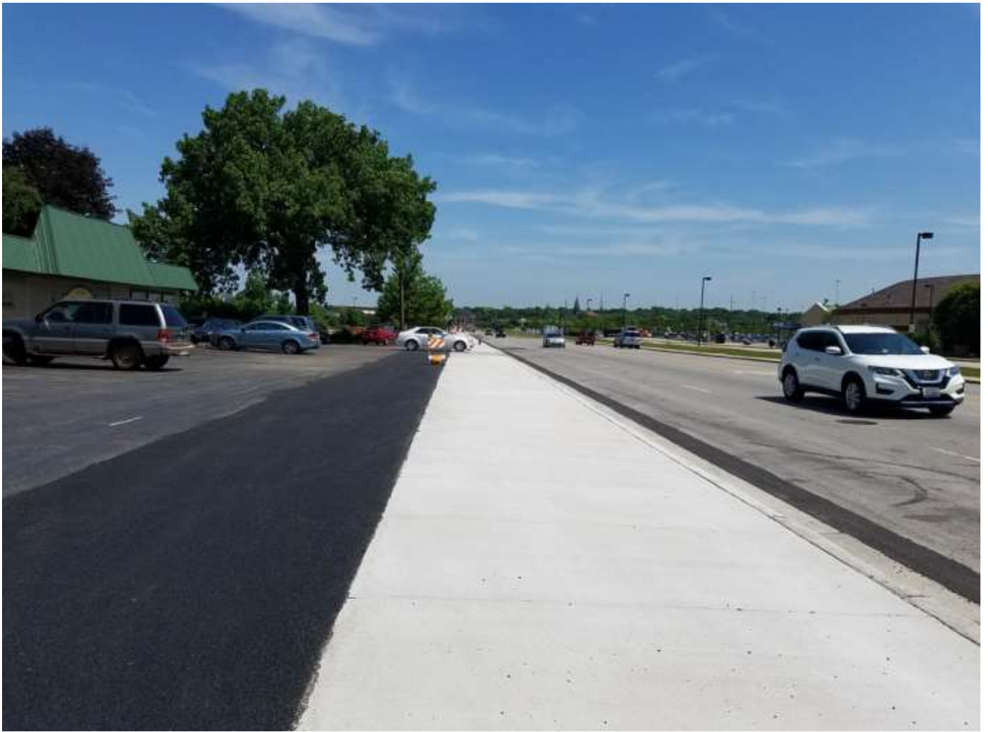
Stage 1- Completion of 10 feet sidewalk along west side of N. Broadway 06/07/2018. Looking north.
