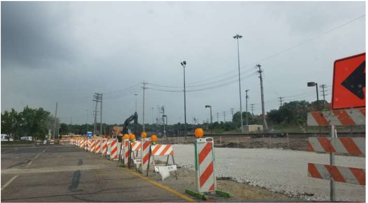
Stage 2- Earth Excavation and Placement of stones along west side of R.R Track. Looking SE.
