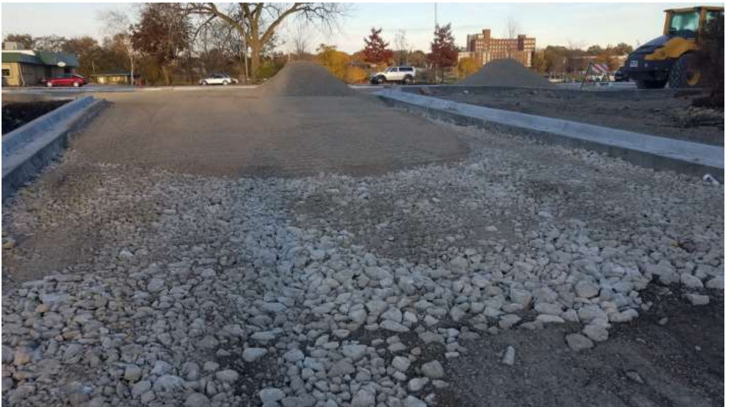
ATC Parking Lot/Pace Staging Area- Looking West- ATC Drive. Placing of capping aggregates. 11/02/2018
