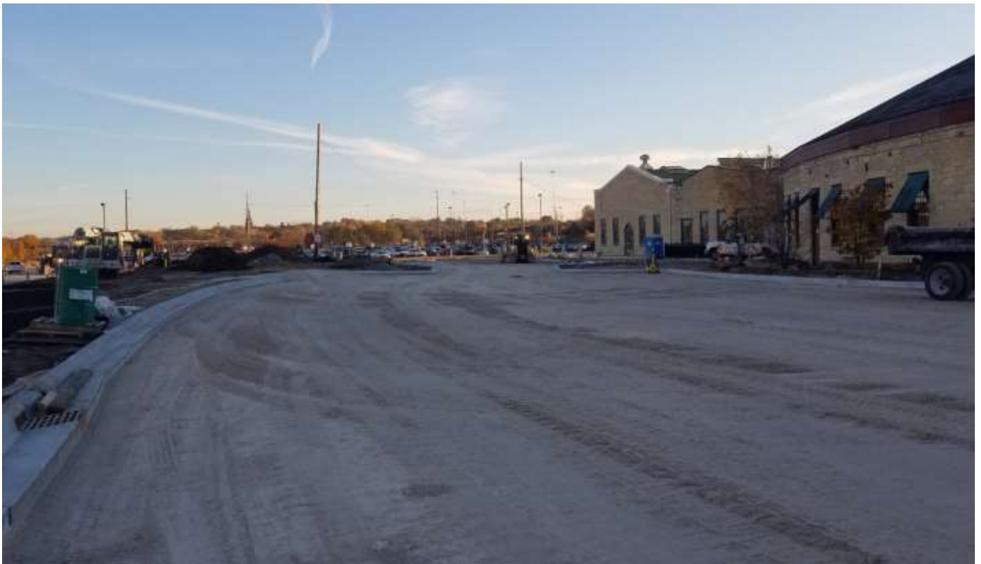
ATC Parking Lot/Pace Staging Area- Looking north. Placing of capping aggregates. Curb and Gutter installed. 11/2/2018
